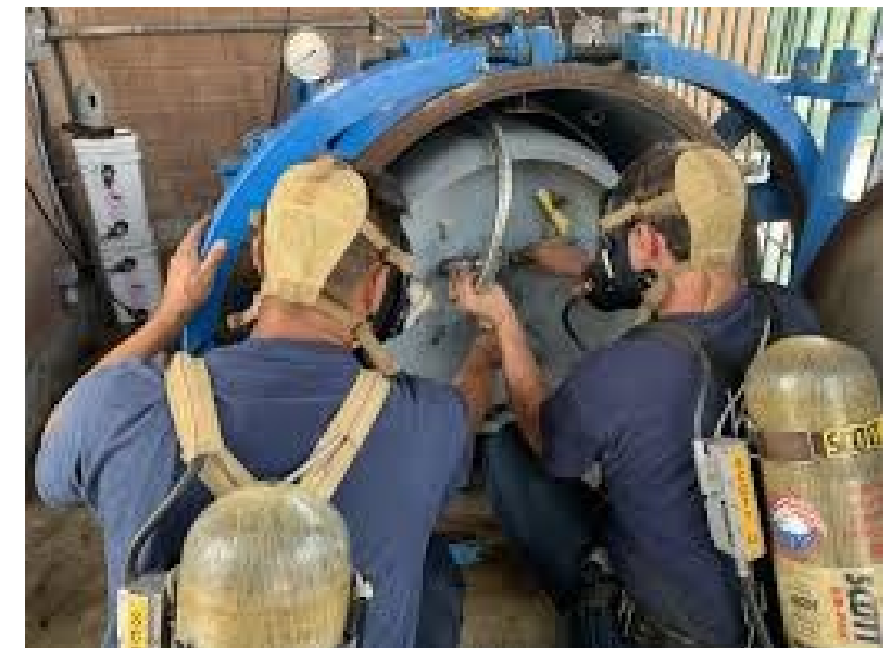
Secondary containment vessel
