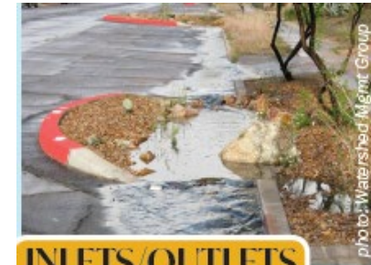
Conveyance allowing stormwater to flow into or out of a GSI feature
