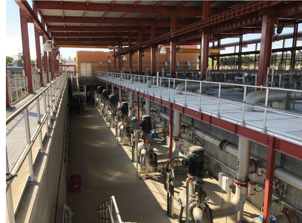
MBR Gallery at Riverside Water Quality Control Plant – CA.
