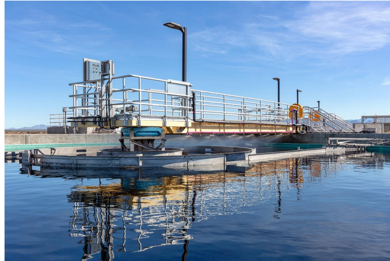
Secondary Clarifier at Marana WRF, Marana – AZ.
