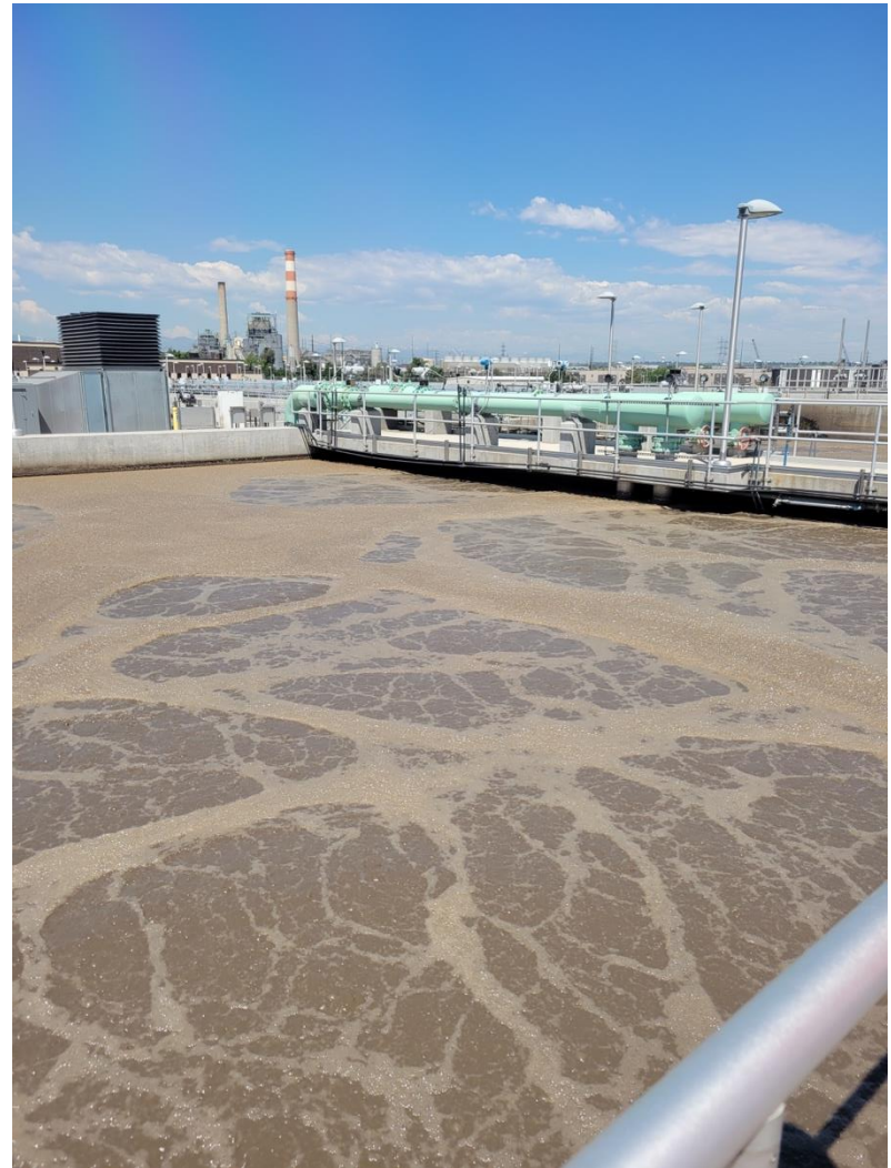
Aeration Tank at Robert W. Hite Water Reclamation Facility, Denver Colorado.
