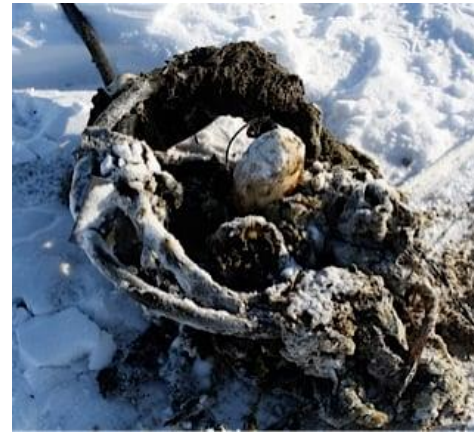
Diffuser clogged with debris
