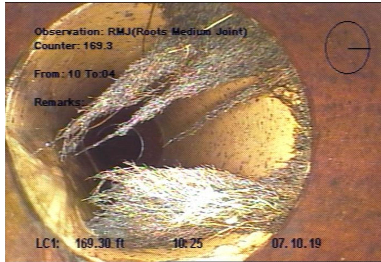
Poor Joint Seal
