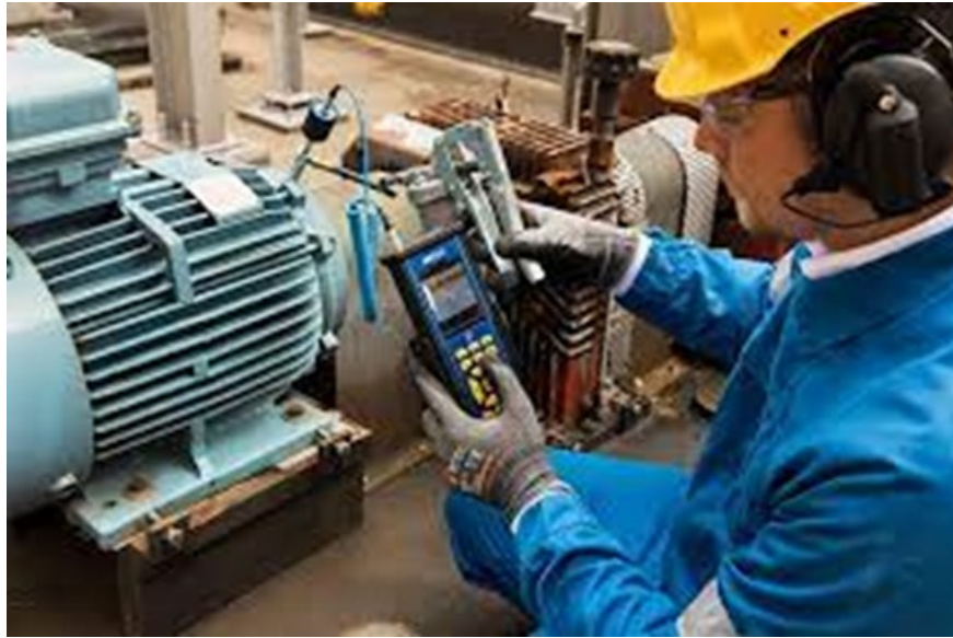
Operator using ultrasound: Increase in noise can indicate impending problems.
