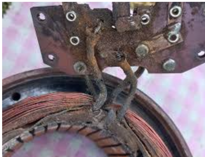
Corroded electrical connections
